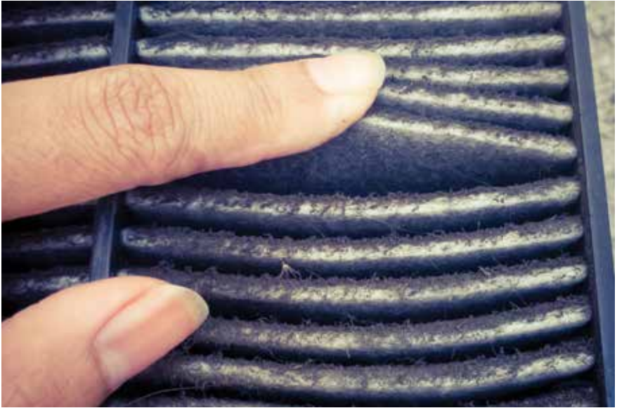
Checking the air filter
