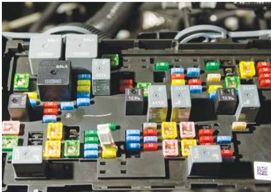
Typical fuse panel
